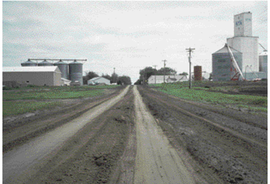
This gravel road shows severe distress after being subjected to a heavy haul from trucks hauling wheat to a grain elevator. The problem was made worse by an unusually wet season.
