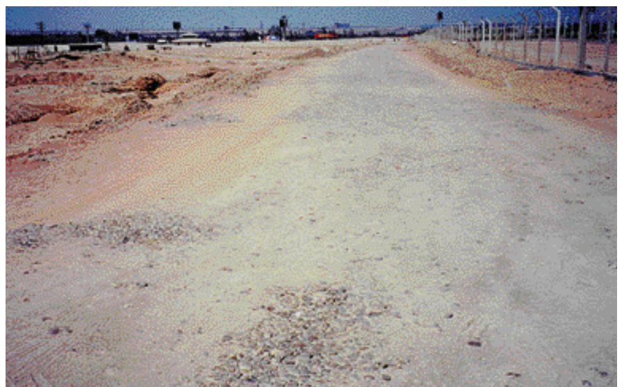
This road is located about 50 miles from Cairo, Egypt. It displays segregation problems in several spots. (Photo courtesy of Ali Selim, SD LTAP, USA)
