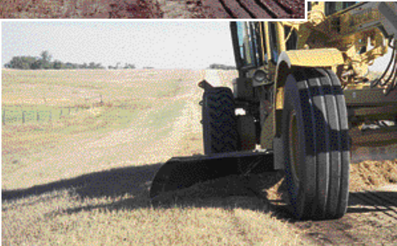
The material from the high shoulder is then pulled into the cut that has just been made. Generally, this material will have to be worked several times with the grader to break it up enough to spread evenly.
